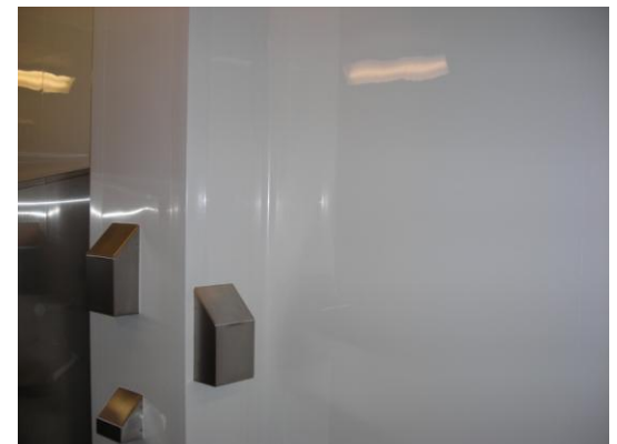
PVC wall panels with stainless- steel shrouded utility ports
