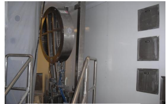
Multiple wall penetrations
